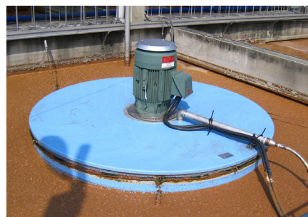
OxyMix installed in a wastewater treatment tank
