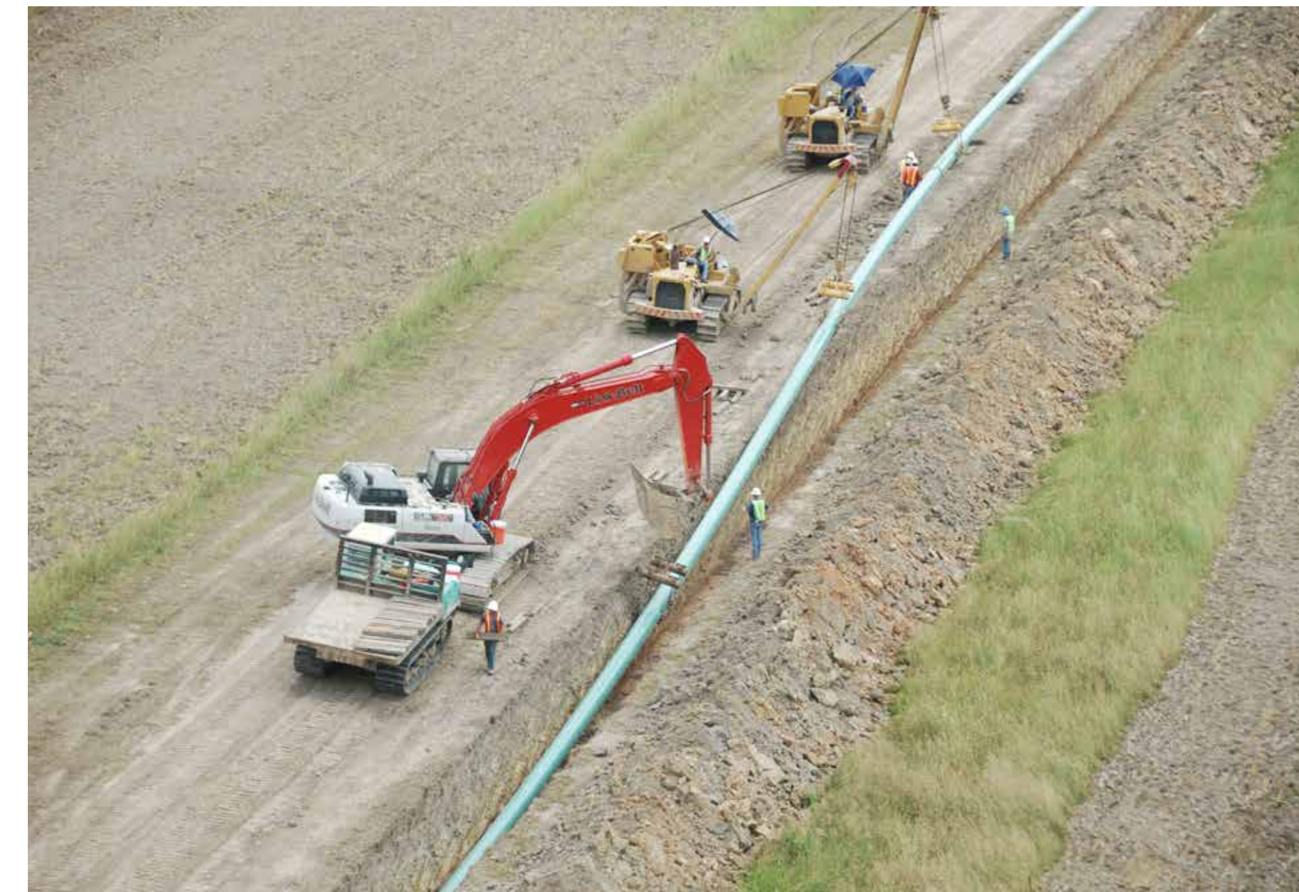
Example of Hydrogen Pipeline
